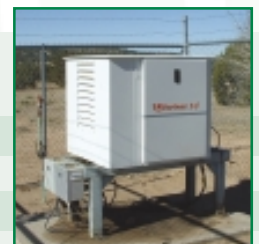
Cathodic Protection On Natural Gas Line – USA
